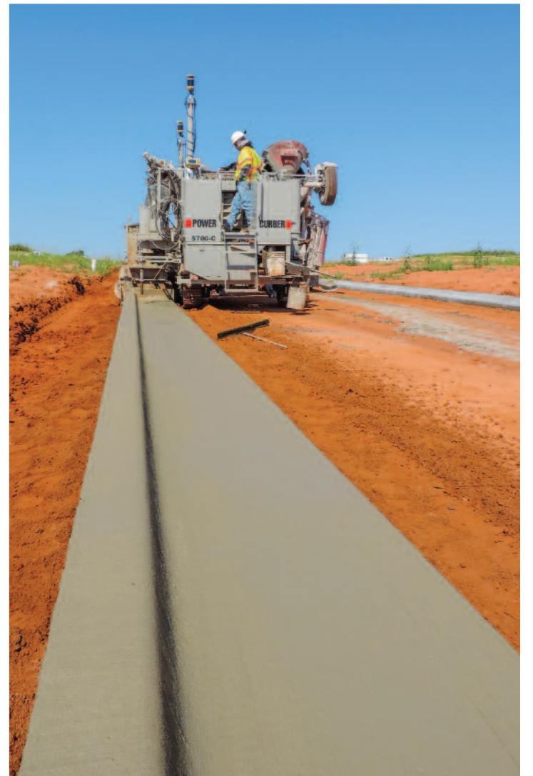
Using the Topcon Millimeter GPS system and a 3D model of the jobsite, Silver Star has eliminated the need to set and remove stringline.
