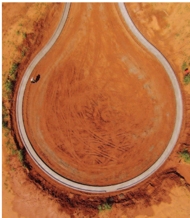
The precision of the curb placement can easily be seen from above.
