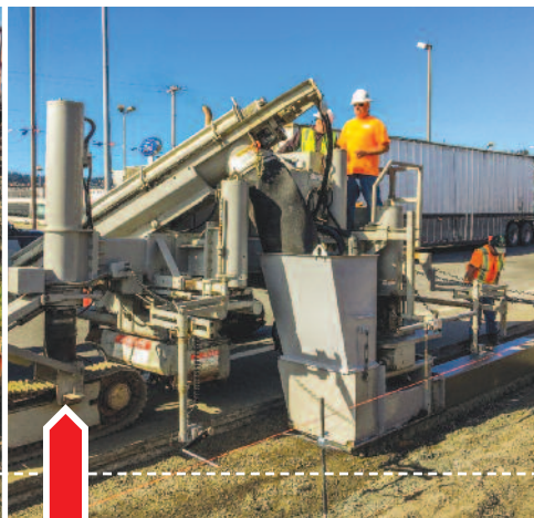
Greg Brock, owner/operator at Brock Construction, realized the value of adding a Power Curber to his business. His 5700-Super-B has already brought in more work for him and his crew.
