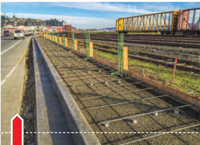
Brock Construction was originally hired to pour the curb and gutter for this project, but once the contractor saw the quality and performance of the Power Curber, he asked them to also pour the sidewalk on the project.
