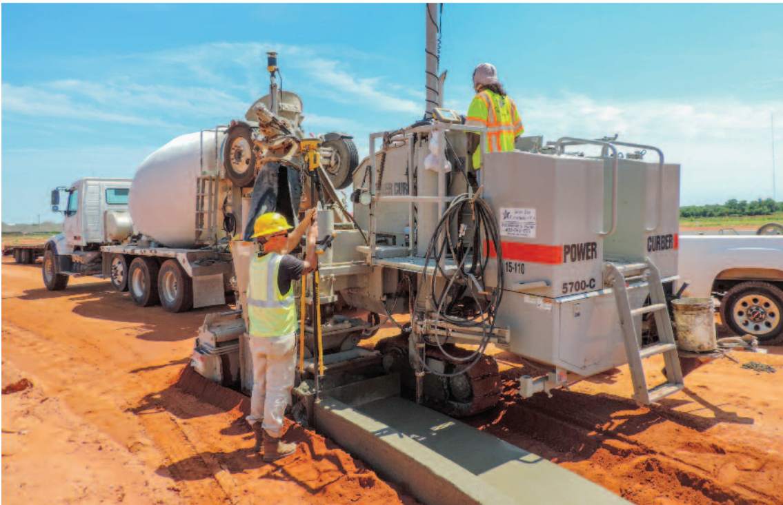
A member of Silver Star's crew uses the Topcon rover to check the accuracy of the curb.
