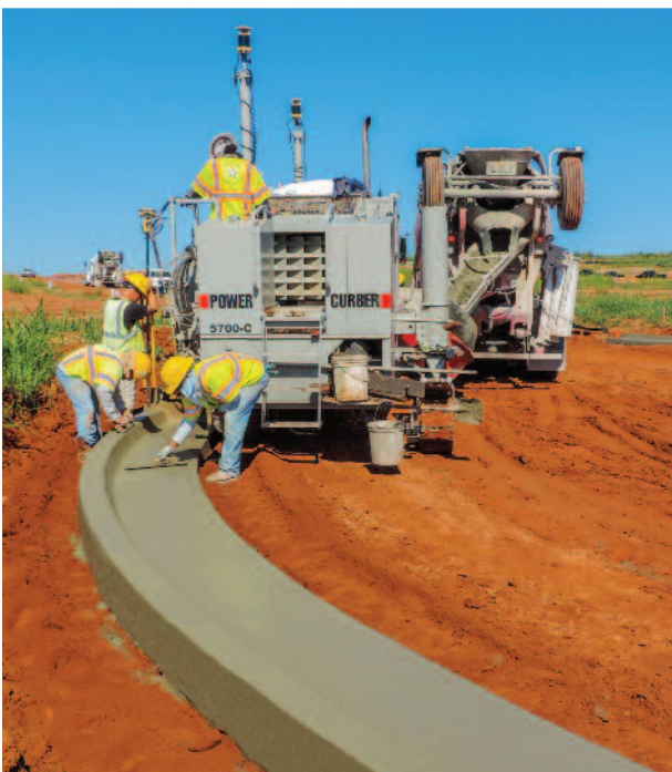
Silver Star's crew uses their 5700-C to pour curb and gutter in a cul-de-sac for a housing addition in Oklahoma City.
