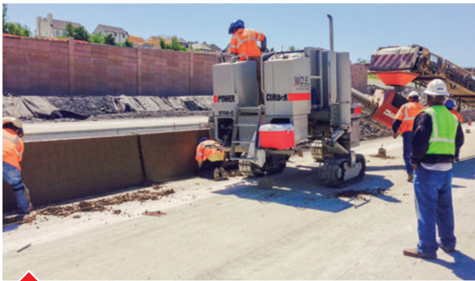
W.O.E. Construction poured nearly 3200 linear feet of colored barrier in one day on the Chisolm Trail Parkway project.
