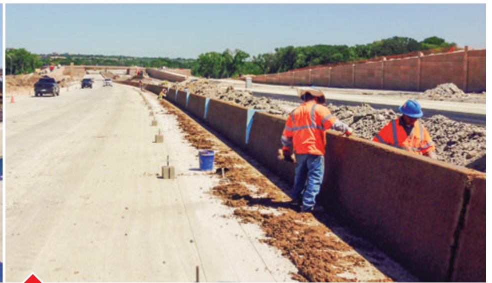
This leg of the Chisolm Trail Parkway runs 26 miles to connect downtown Fort Worth, TX, to the suburb of Cleburne.
