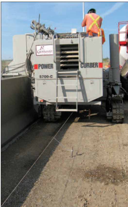
A second stringline is under the machine to control the variable side of the barrier mold
