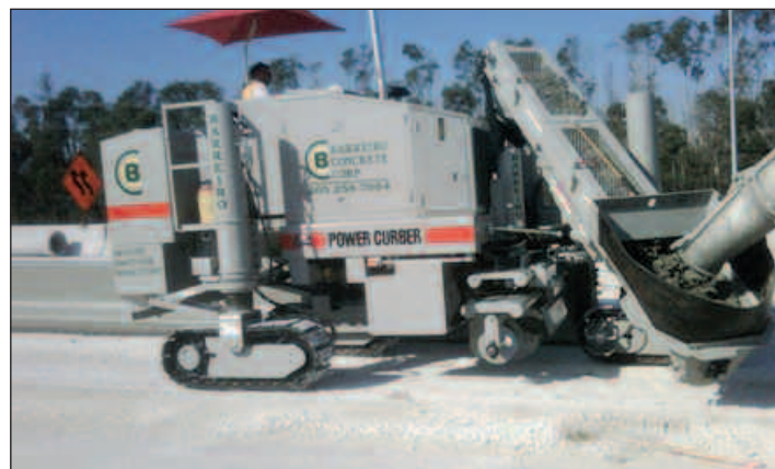
The optional Trough Top Auger Conveyor, Weight Pod, and Polyurethane Track Pads enhance the machine for barrier work. This 5700-C is owned by Barreiro Concrete of Princeton, FL.
