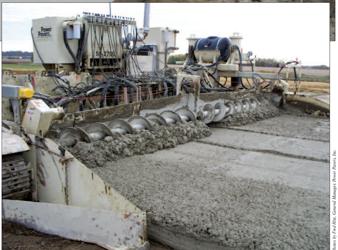
The concrete is supplied in front of the paver with a Power Pavers PS-2700 Placer/Spreader to ensure a consistent supply.
