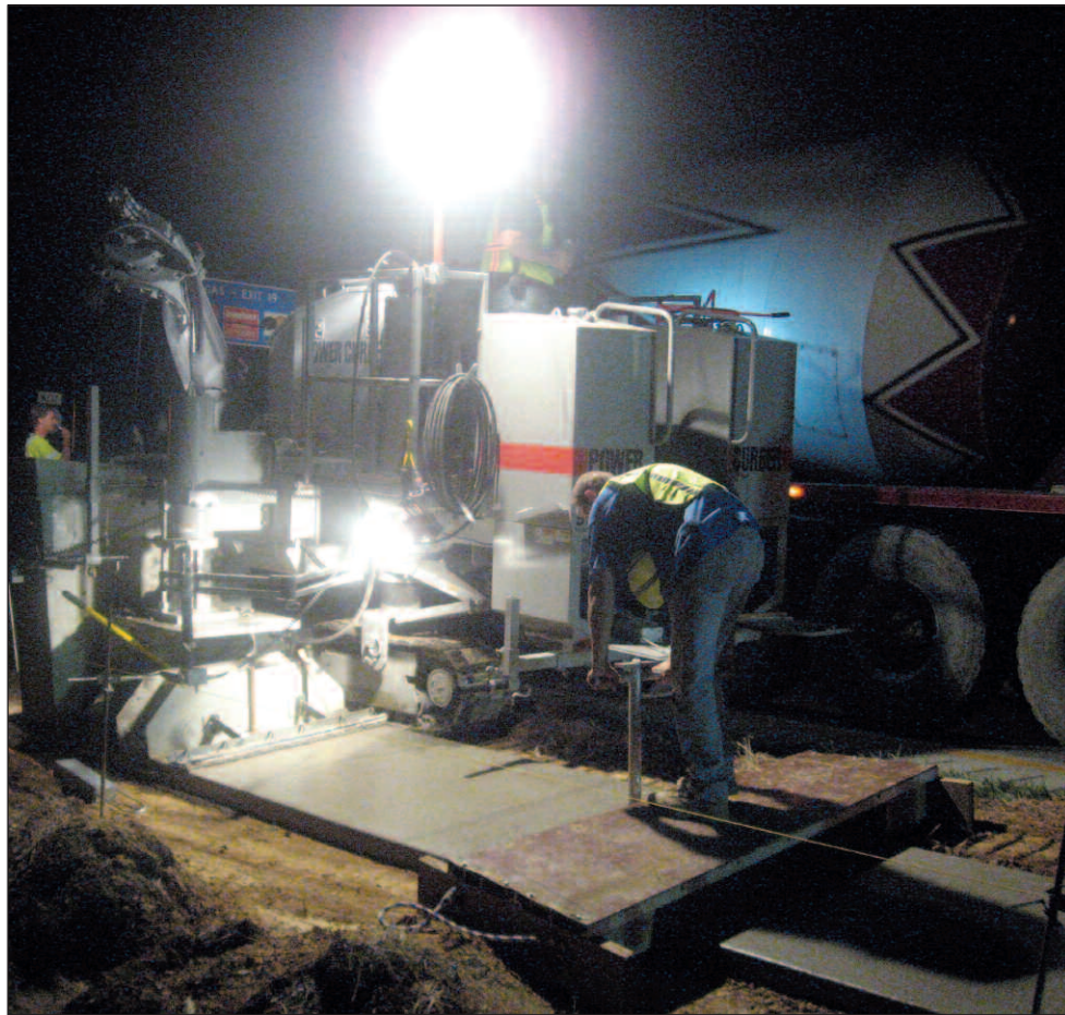
Machine pours foundation, while crew sets anchors for posts in fresh concrete
