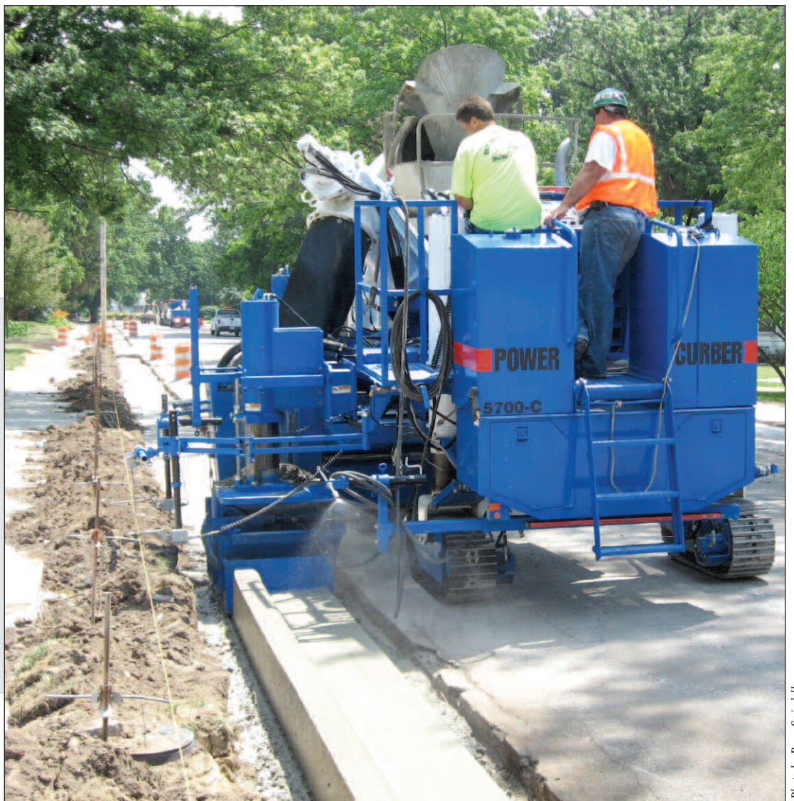
CC & T of Indianapolis finds high spots in the asphalt are no problem in rehab work with the 5700-C
