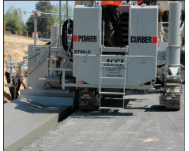
Atlantic Contracting Co. of Greensboro, NC, poured this 48-inch wide (122cm) highway shoulder with its new 5700-C.
