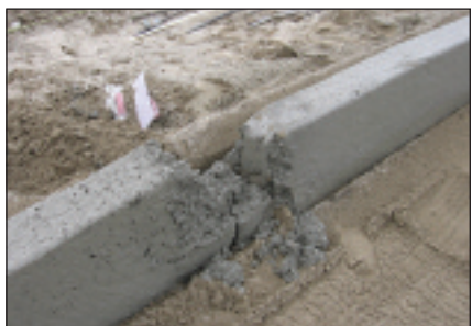
Curb Appeal's work represents very little tie-in work in parking lot islands
