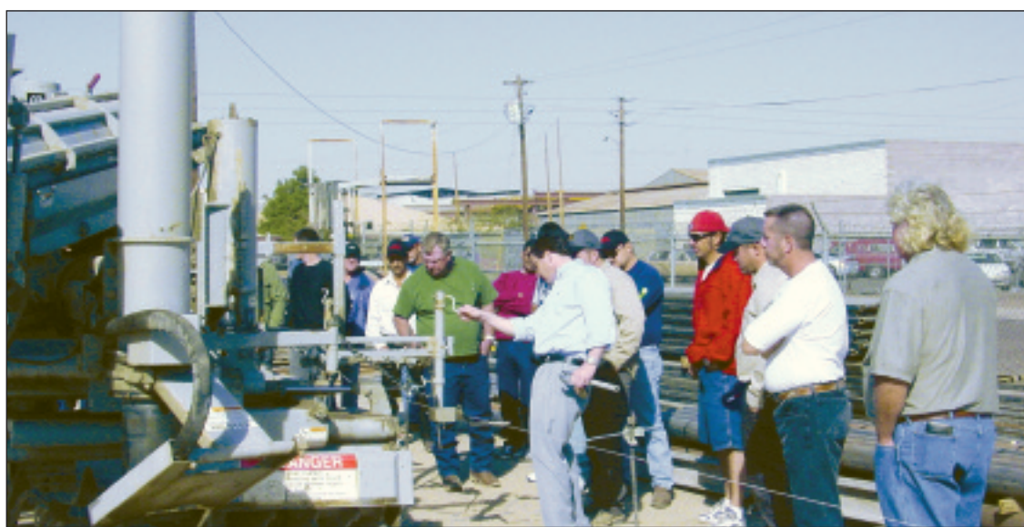
Power Curbers technician Brandon Bello, center, turns jack handle to adjust sensor wand in discussion on stringline at a hands-on class in Phoenix
