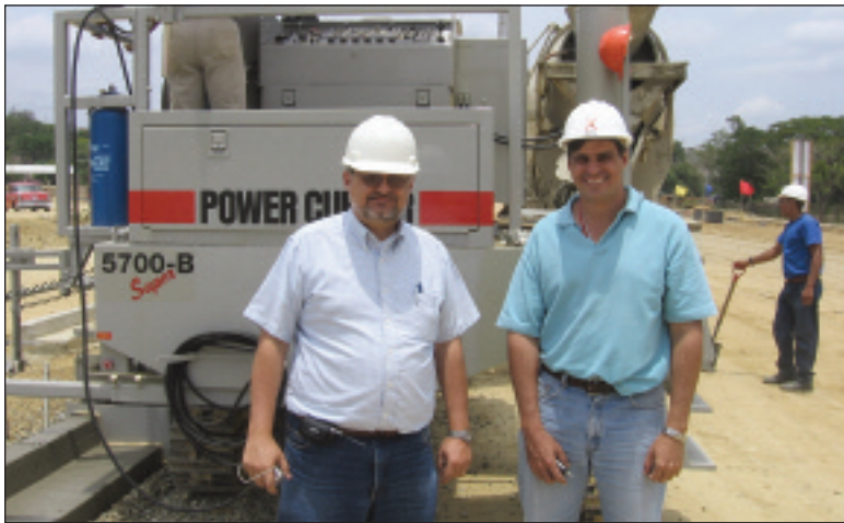
Pedro Azpurua, Inc., left, and Roberto Cavallin of Consorcio Pueblo needed the 5700-SUPER-B to install 55 kilometers (34 miles) of curb
