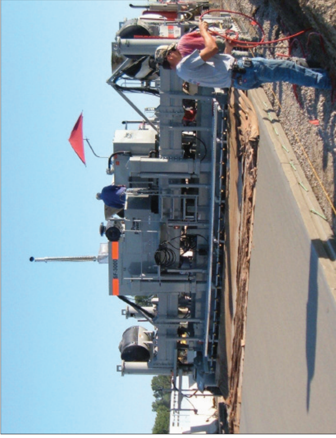
Sioux City Engineering of Sioux City, IA, paving 24 feet wide (7.3m), 10 inches thickness (25cm) with SF-3000. Steel female keyways are being inserted in the center of the slab and will tie into the next lane to lock the lanes together
