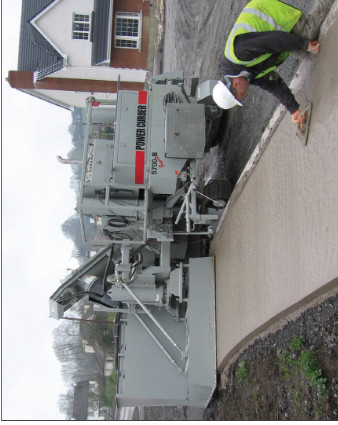
6-foot (1.9m) sidewalk: 'It would have been a lot more expensive by hand,' says contractor
