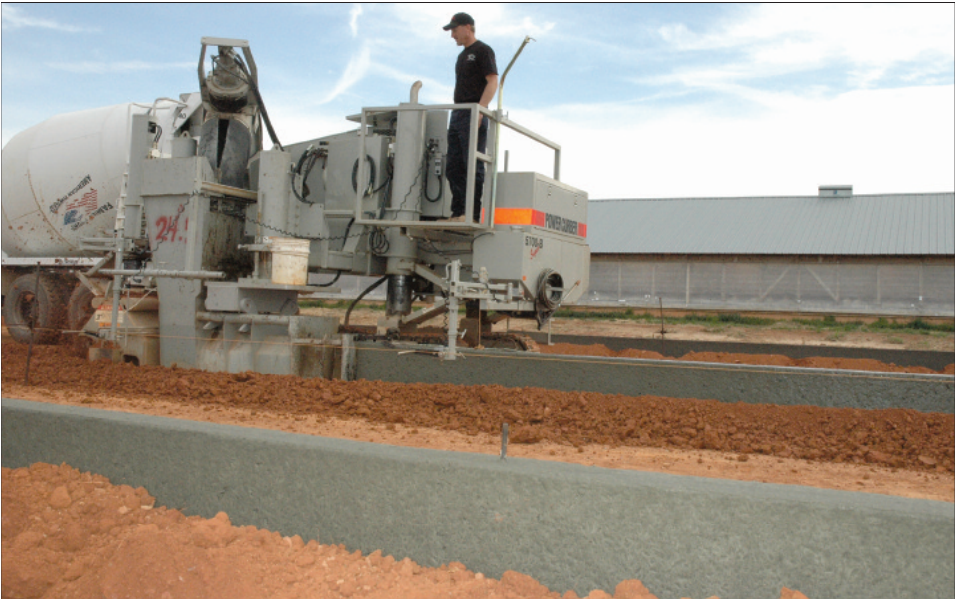
Machine operator Chuck Witfield, shown here pouring a foundation for a second chicken house at a farm in Lavonia, GA, says that foundation work is harder than curb work. The wall has to be exactly right, he says — straight and flat across the top for the framing
