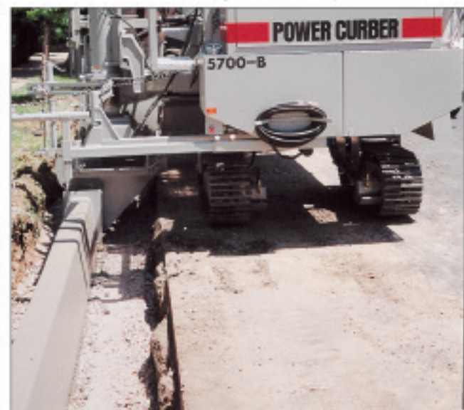
In this rehab application involving 18-inch curb (45.7 cm) in New York, the base of curb is 14 inches (35.5cm) below grade and 18 inches (45.7cm) from the edge of pavement.
