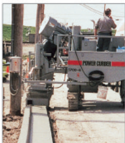
The back of curb passes within inches of the utility pole in this rehab job in Indiana.
