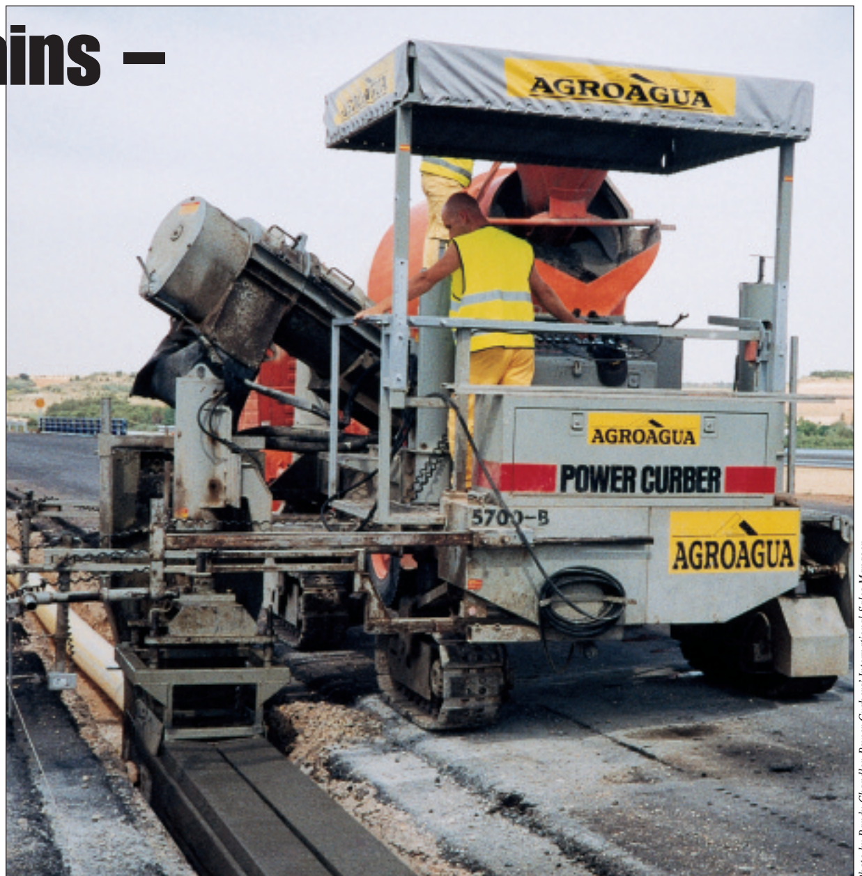
Inflated plastic pipe is removed after concrete hardens, leaving cylinder for water runoff
