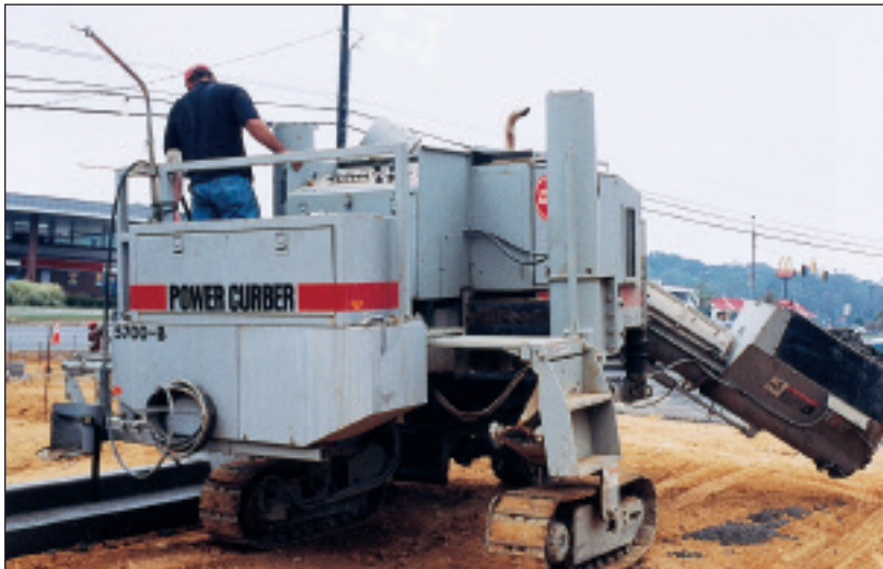
Fernando Rodriguez gets curb on the ground — the machine has resulted in a big increase in work
