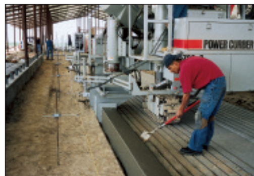
The machine slipforms a 12-inch tall (30cm) water barrier in the 'flushing lane' that will keep water out of the sleeping stalls
