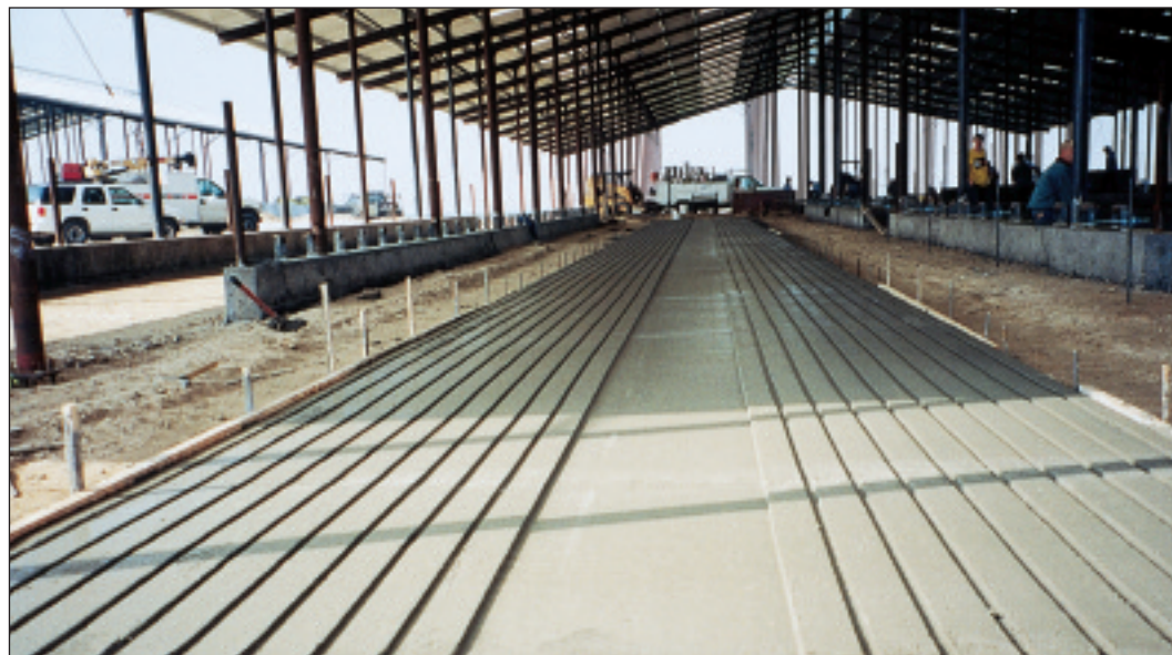
This 'flushing lane' in the center of the barn is being installed with 5 different pours of the machine, including this 10-foot center-pour application (3m). The 24-inch wide (61 cm) smooth area in the center of the slab is 5/8-inch deep (1.58 cm). A mat will be placed in it and it will be used for a walkway. The grooves installed by the mold on either side of the walkway are an inch apart and 1/2 inch deep (2.5 cm apart and 1.27 cm deep). These areas will be used to wash away waste. Two 5-foot wide sloped bedding stalls (1.5m) will be slipformed on either side of the slab
