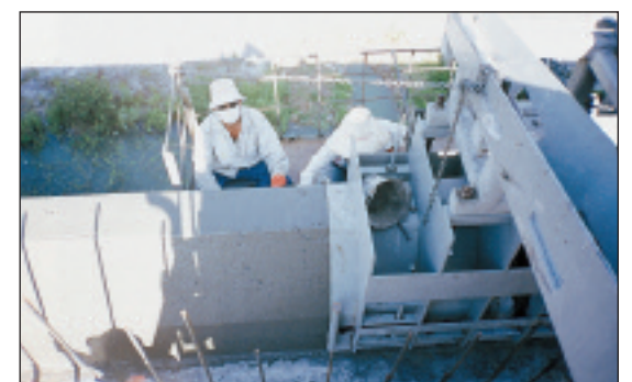
The upstream face features a graduated change in the slope (top photo). As the dam moves toward its planned height of 93 m (305 feet), the upstream face becomes vertical. The dam was 55 m (180 feet) in the air when these photos were taken. Finishers (lower photo) work from a basket suspended over the side of the wall and attached to the mold
