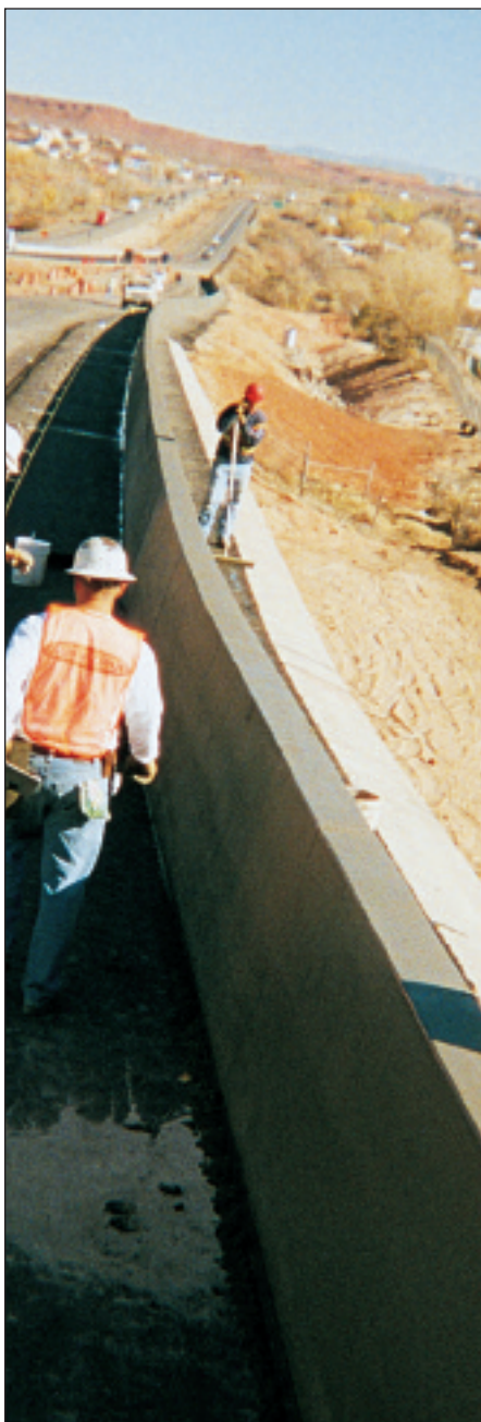
Photo shows the coping application (right) atop the Mechanically Stabilized Earth (MSE) wall and the constant-slope parapet (center). Both applications were slipformed with the 5700-B
