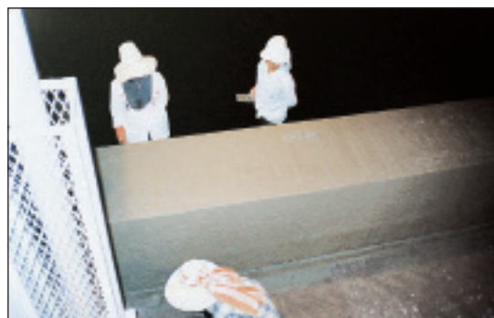
The downstream face (top photo) is stepped. The interlocking passes vary in width from .3 m (.98 feet) to .7 m (2.29 feet) and in height from .6 m (1.9 feet) to .9 m (2.9 feet). Finishers (lower photo) stand on the steps to work on the outside of the wall
