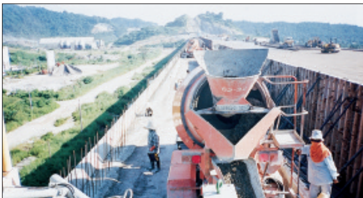
This photo shows a portion of the walk-through gallery being constructed between the upstream and downstream faces. When complete, the dam will rise to the crest of the hill shown in the background
