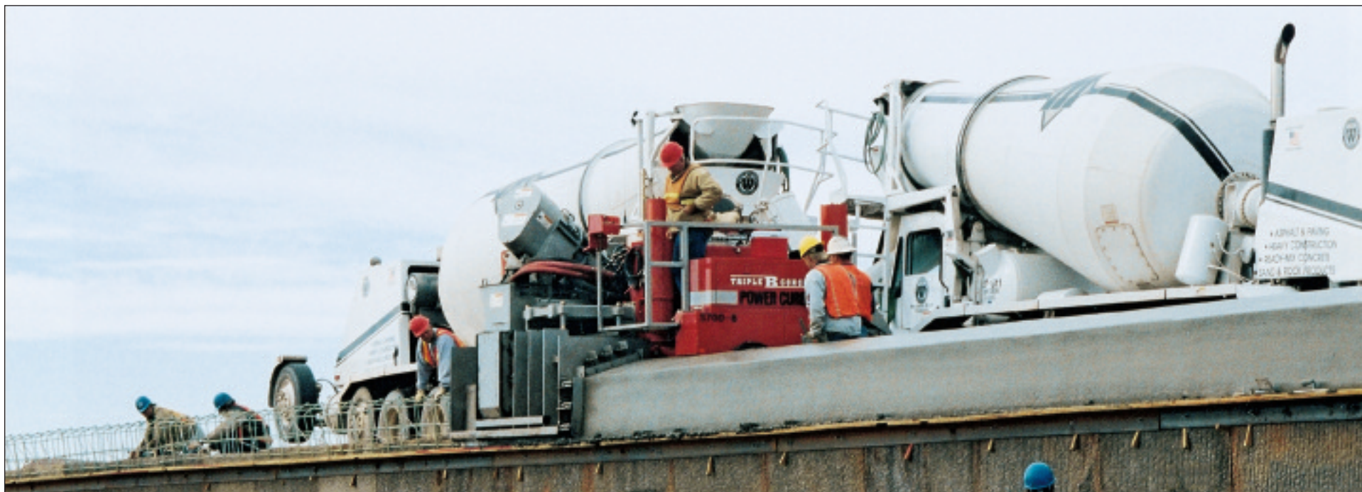
Slipforming the coping, a 2-foot by 2-foot block of concrete (.6 by .6m) on the bridge, was a big deal for state DOT officials and the general contractor. This was going to make or break the job, says Brant Anderson of Triple B Concrete of Cedar City, UT
