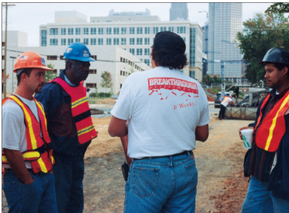
Everett Martinez, center, superintendent of Crowder Construction Co.'s curb crew, walks the job with his crew before the pour begins. It's part of the 'Break Through Performance' Program that
