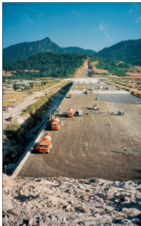
The dam is being slipformed in sections, between the rugged terrain of Nakorn Nayok Province
