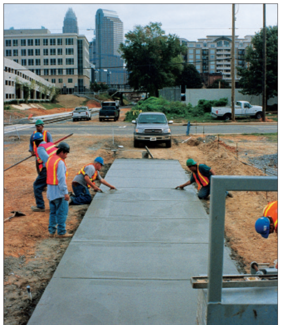
The walking path runs parallel to the rail (seen to the left of the pour) that will be used by trains and trolleys to move people from events in downtown Charlotte, NC, to condos, clubs and restaurants in the south end of the city
